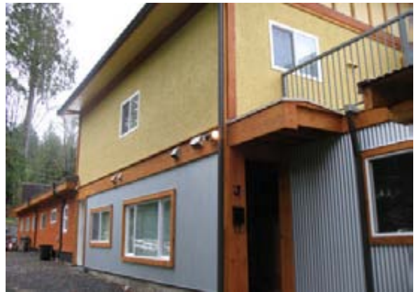
Unit J, completed by November 1st, exemplifies recycling and design practices at UEP by providing an attractive and comfortable interior for an affordable price ($600+util) - while using recycled cabinetry, appliances, trim materials and doors.
